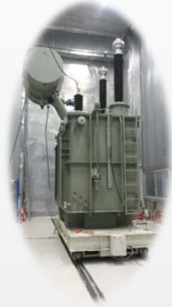
25 MVA 154/27,5 kV MONOFAZE, TCDD PROJESİ
